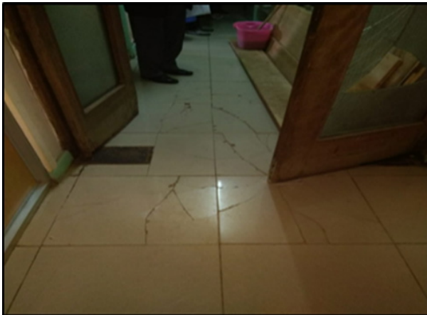
FIGURE 1 Broken floor tiles at Works Building Source: Field study, 2026
