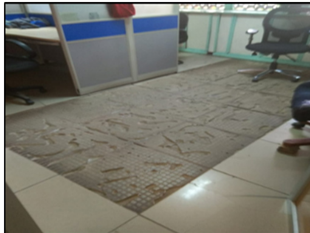
FIGURE 2 Dilapidated floor at Works Building Source: Field study, 2026
